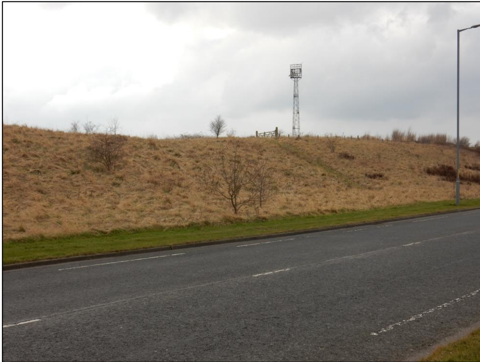
Plate 34. The cycle lane paintwork has worn away on the road. The embankment on the opposite side of the road is the site of the 1830 trackbed and has a desire line up to the gate which leads to a biomass regeneration site, but also a well-used path affording views of the rail track. This embankment continues until just short of Thornaby Station.
